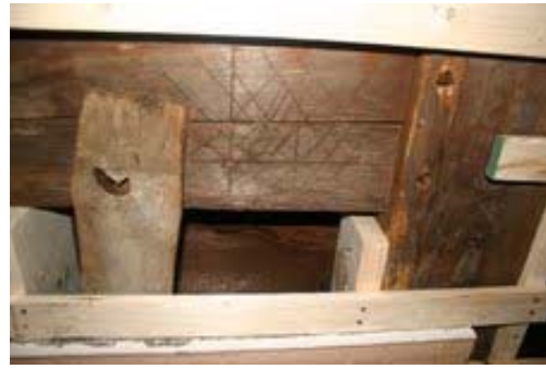
A view of some of the original Devotion House beams with new support in place.
